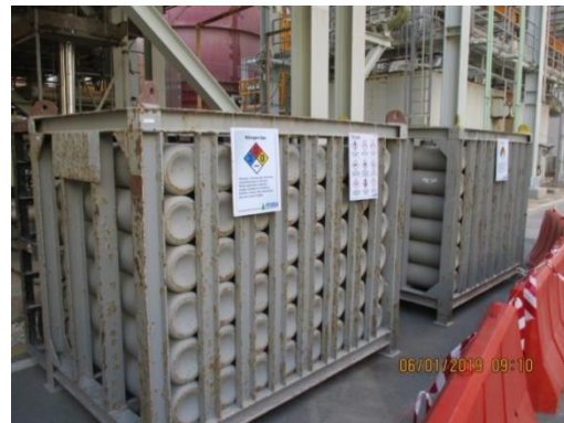
Compressed gas cylinder storage in cage with Signboards and barricades
